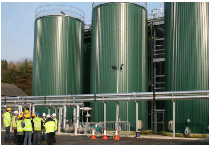
A recently commissioned anaerobic digestion facility
